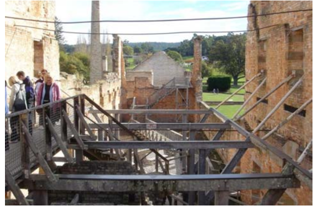
What is left of the building, structural support to keep the walls from collapsing.
